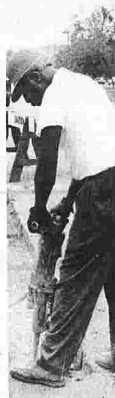
Workman for R. Aleria & Sons drills for new curbing at E. Center and Spruce Sts.
