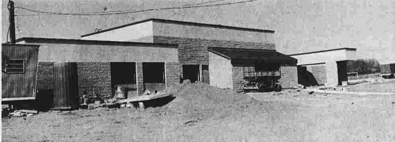
This is the Regional Occupational Training Center nearing completion. It will open in the fall.
