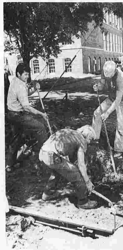
Public works department engineers lay sidewalks from Main St. to the side of the church near Lincoln Center.
