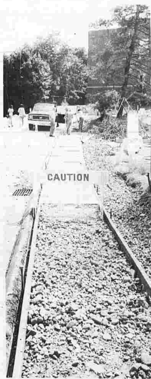
Town engineering department people construct sidewalks along rear of Municipal Building parking lot to Lincoln Center in the background.
