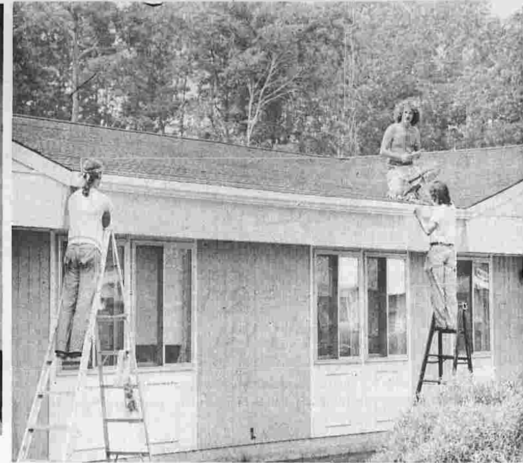
Bob Woodward, left, "Kip" Toss on the roof and Mike Tuthill install gutters at a building at Manchester Community College.
