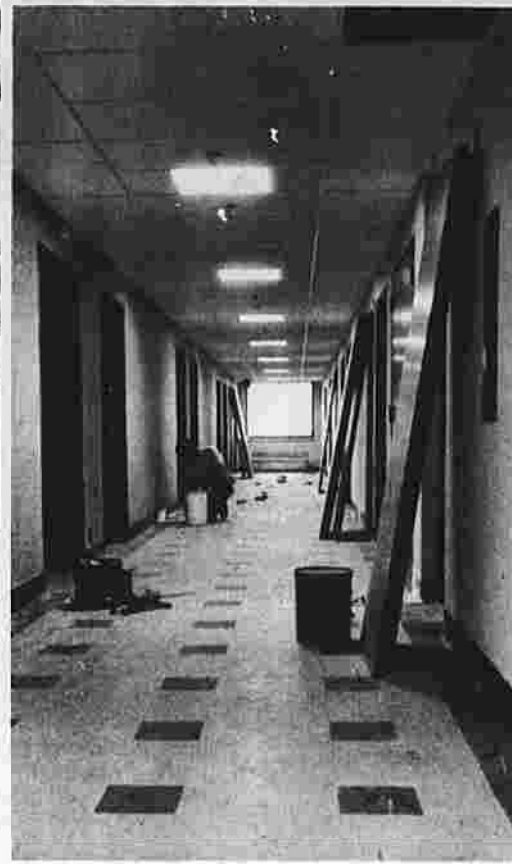
A workman spreads a sealing compound in preparation for applying baseboard in a corridor at the North Wing of Manchester Memorial Hospital.
